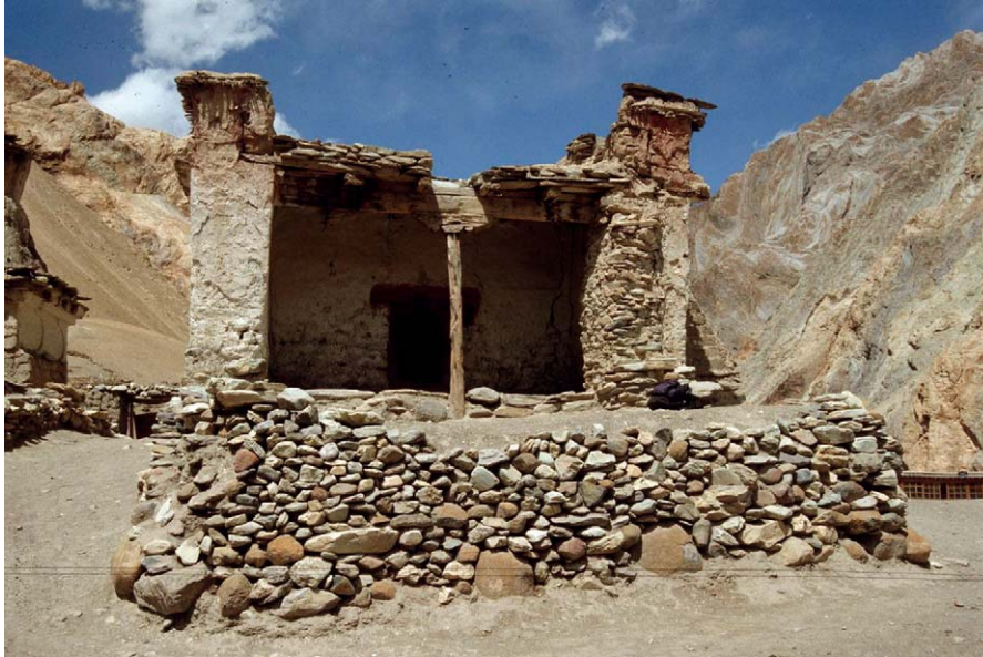
Fig. 1: The Lo tsa ba lha khañ as seen from the south (© Christian Luczanits, WHAV, CL 00 44,39)
