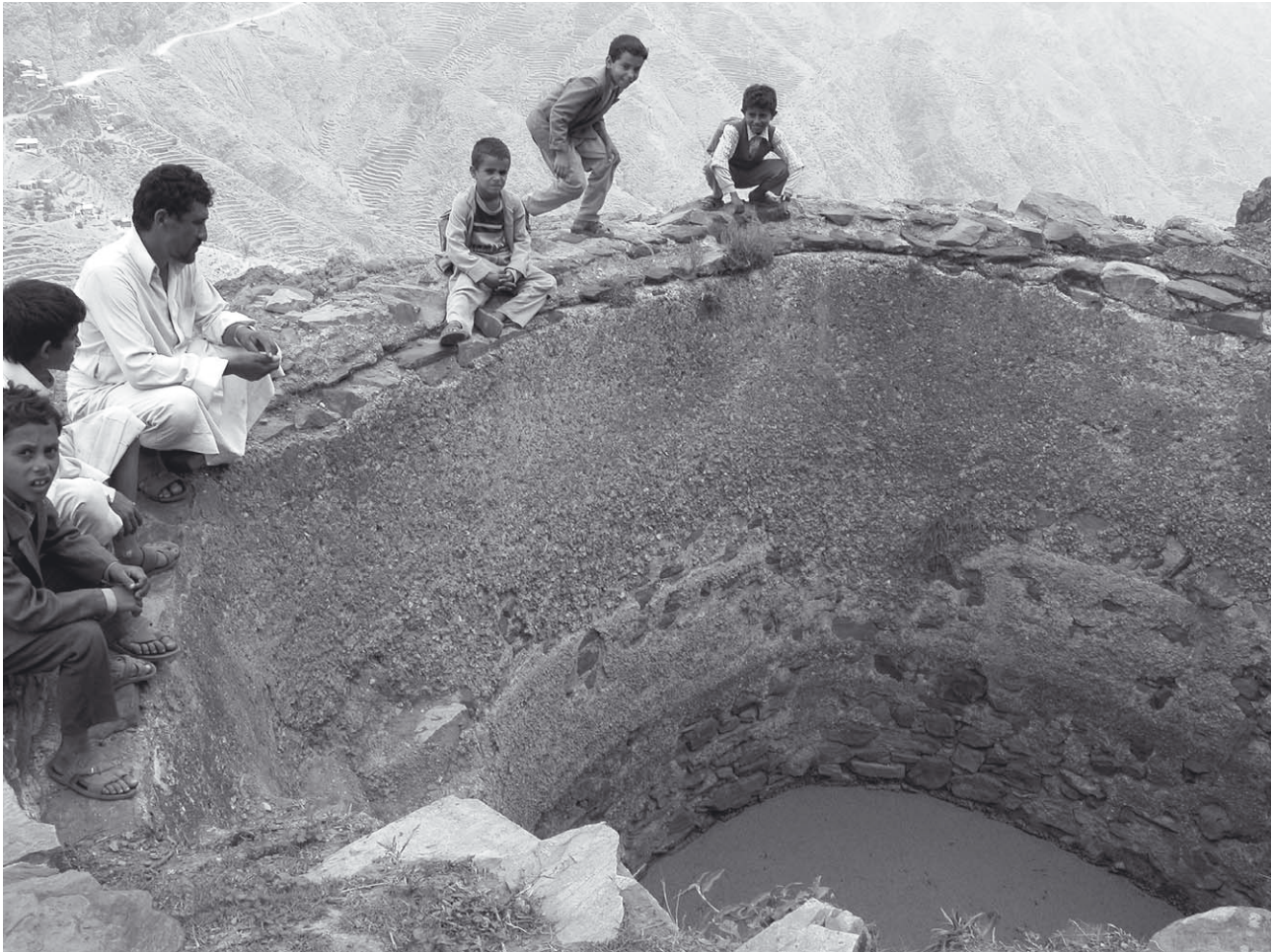
Figure 3: This is an old cistern where one can easily see how the qaḍāḍ has worn away near the bottom. The cistern was leaking and in need of re-plastering. (Photo: E. Hovden)
