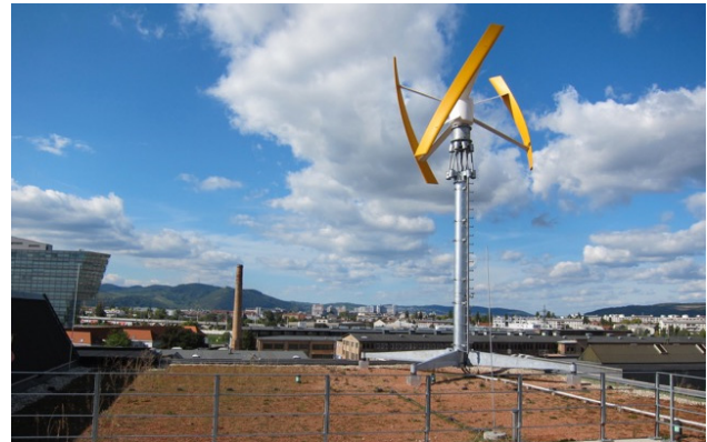
Urban wind turbine integrated in the building
