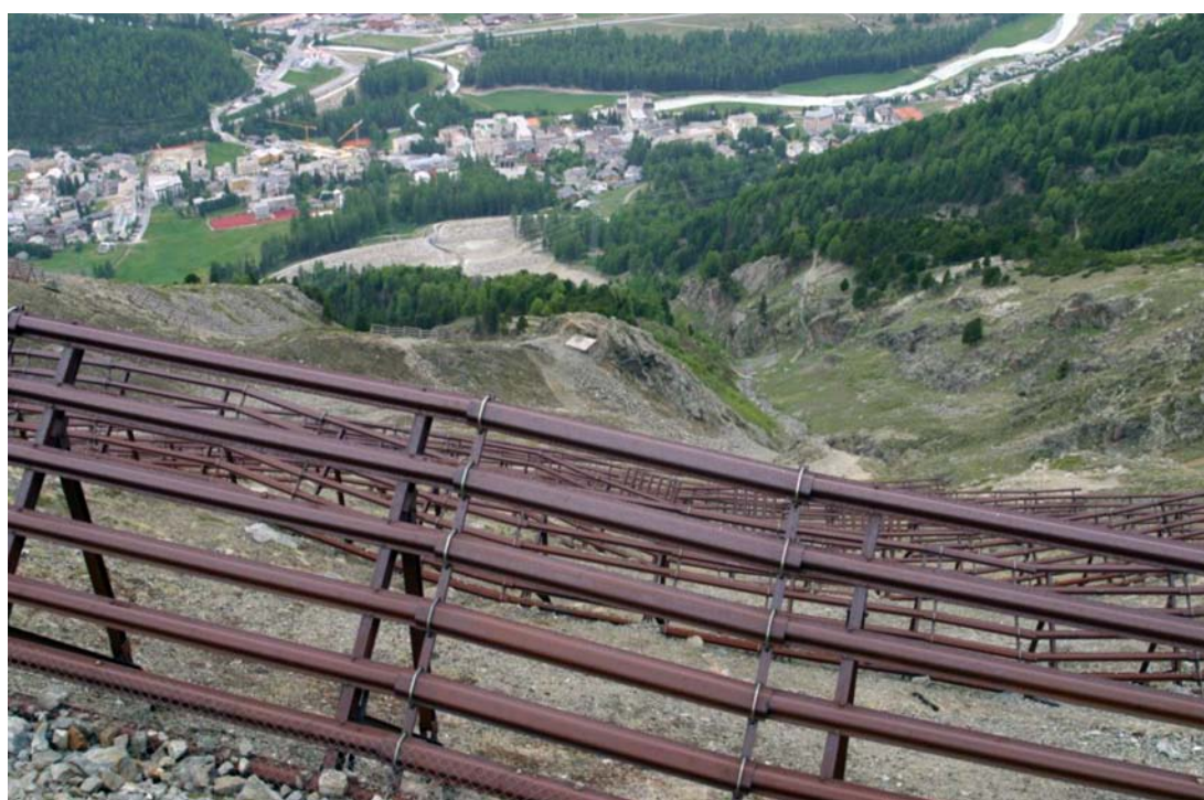
Fig. 2: Avalanche and Debris Flow Protection Above Pontresina, Engadine Valley, Switzerland.
