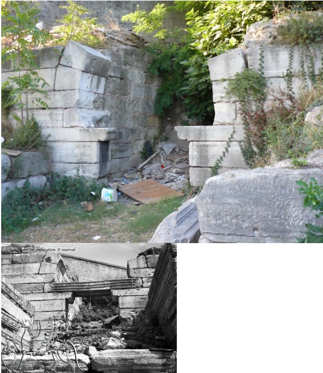
Fig. 7 Gate by the Boukoleon palace, with broken inscription in tabula ansata . State on 5/9/2018, and the old restoration of the block by Mamboury (© DAI Istanbul archive)
