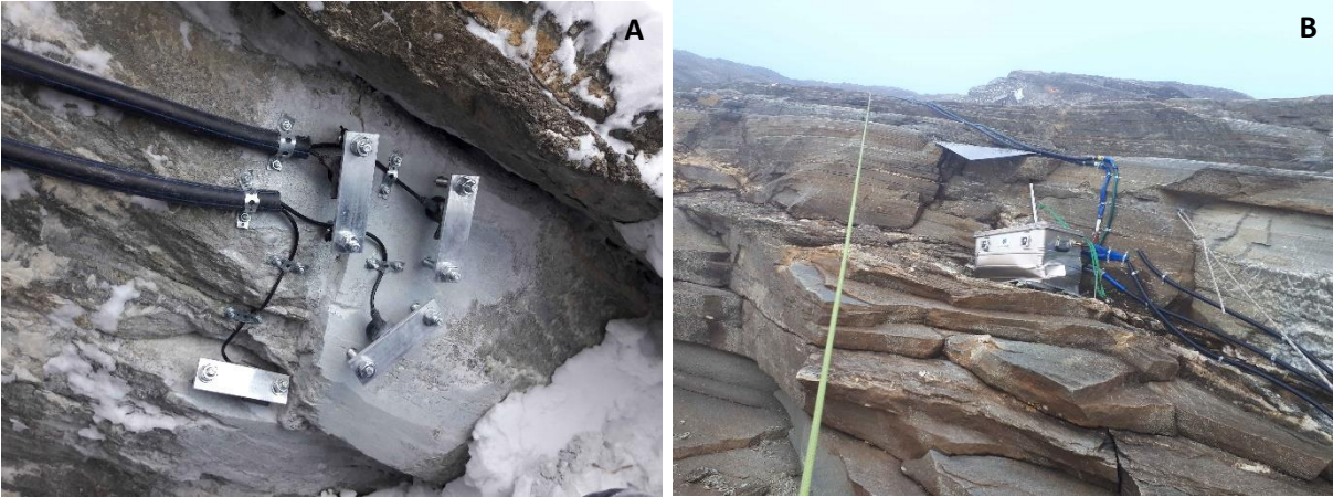
Figure 20: (A) Acoustic emission (AE) sensors (Mistras R6I-UC Sensor) installed directly at the randkluft opening (MS Randkluft Lip); (B) Aluminum box immediately above the AE monitoring twisted by snow pressure.
